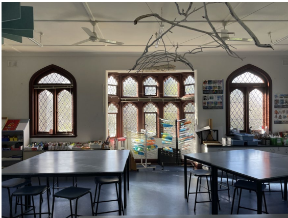
Figure 13. Oriel windows to first floor. Embedded steel elements forming lintels over the window openings show visible evidence of corrosion which is causing cracking in the surrounding concrete. (Image: Urbis June 2023)
