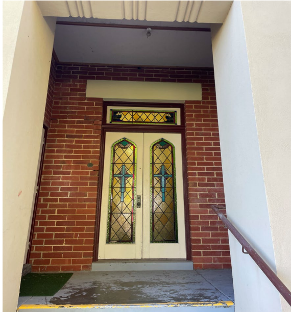
Figure 15. Leadlight detailing to side entrance to southern wing (c1940). (Image: Urbis June 2023)
