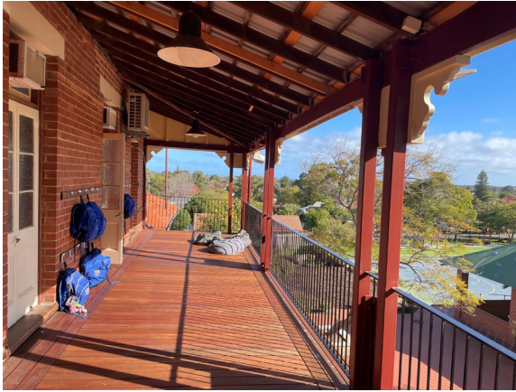
Figure 8. First floor verandah to northern wing (1931) showing repairs undertaken in 2021 including replacement steel posts and decorative brackets and valances. (Image: Urbis June 2023)
