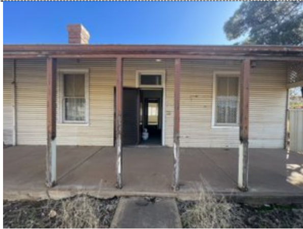
Figure 14. East tenancy entry and modified posts
