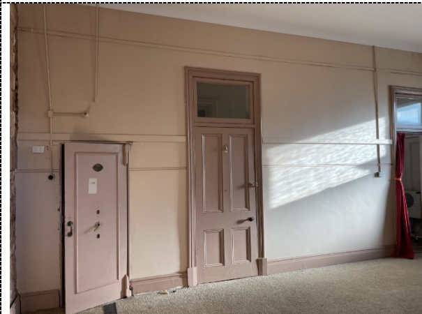
Figure 40. Former GWS Office - Safe and Door
