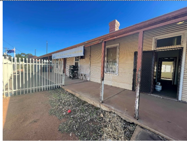
Figure 16. View of fence diving east and west tenancies of the Police Station
