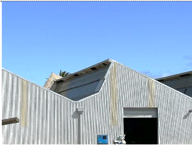
Figure 17. The glazed panelling to the southern side of the roof form and truck entry into the warehouse.
