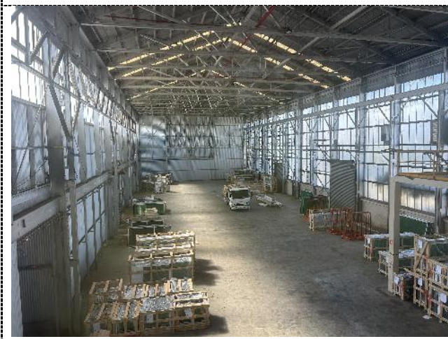
Figure 28. Southern warehouse, taken from the upper offices. The trusses are timber in the original section, while steel trusses have been used in the later addition. The timber trusses have been painted silver.
