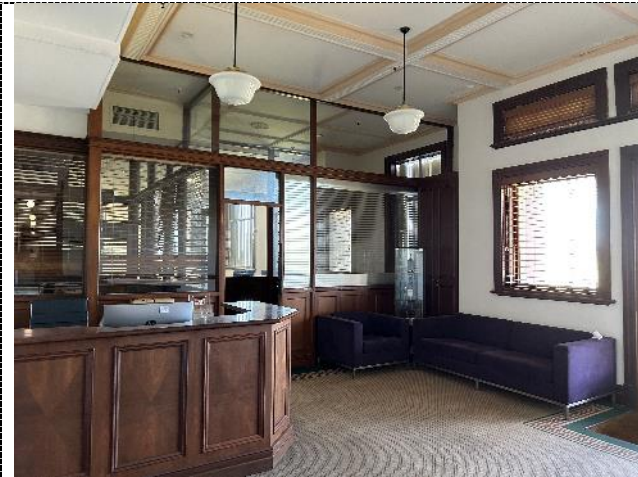
Figure 20. Reception/display area. The reception desk is not original although has been constructed to reflect the original timber partitioning of the offices. The ceiling is original.
