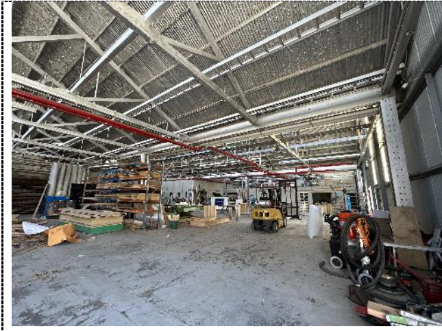
Figure 31. Saw tooth roof warehouse. The remaining warehouse bays date to the original 1930 construction, with timber trusses throughout. The timber has been painted silver.
