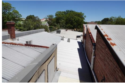
Figure 15. View from Manager's Residence window – showing form of sawtooth roof, chimney to single-storey Residence, and two high-level west facing windows (now boarded over) that lit rear of Adjoining Shop. Skillion roof next to chimney illustrates width of original residence. Continuation of skillion at slightly shallower pitch illustrates area of former courtyard that was enclosed and redeveloped c.2010-2011. 58
