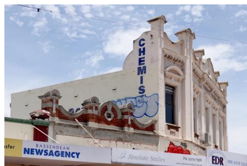
Figure 13. Parapet detailing of single-storey shop largely intact. Removal of paint revealed original brick and stucco.
