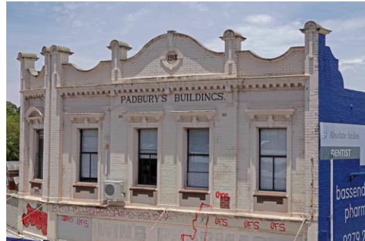
Figure 9. Façade originally face brick with contrasting stucco detailing now painted. Original multi-paned sash windows replaced with aluminium-framed windows. High-level windows to the shop (above awning) boarded up. Most of the decorative detailing has been retained.
