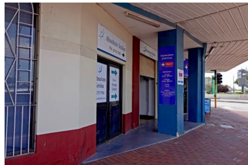
Figure 11. Original frontage to stairwell followed approximate line of concrete paving. Free-standing columns support original line of first-floor facade. Panelled timber door with multi-pane fanlight windows, which formed recessed entry of original frontage, replaced by metal roller door at new setback.
