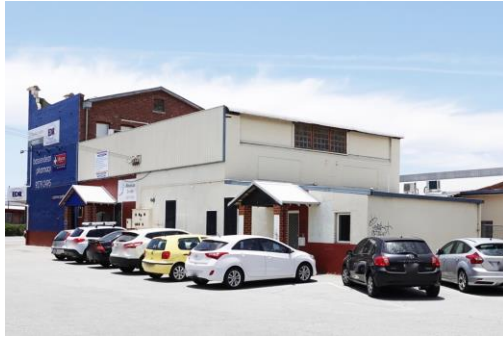
Figure 14. Saw-tooth roof of single-storey section concealed behind flat-pan metal parapet. Section of multi-paned saw-tooth windows still visible at south end. High-level windows to original south wall (now boarded over) can be seen. 57 Original face brick walls, timber-framed sash windows, and louvred gable vent to rear of Manager's Residence still visible. Rear skillion c.1960. Doors and windows along west elevation from rear of the shop and two portico entries c.2008.
