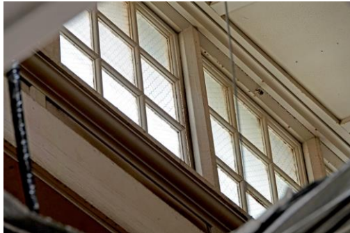
Figure 16. Original detailing of multi-pane sawtooth roof windows visible through open skylight hatch to east-west entry passage off carpark. Small section of former high-level panel and batten ceiling also visible.
