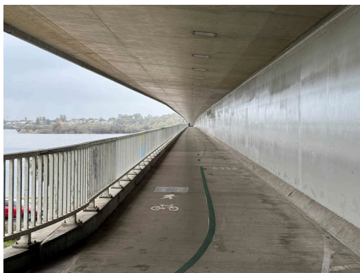
Figure 6: Mount Henry Bridge , from west side, showing shared pedestrian and cycle footway, cantilevered under the road bridge.
