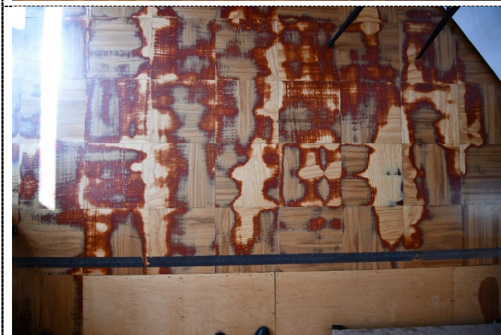
Figure 43. Original Boardroom parquetry flooring has been damaged by past tenants trying to remove timber staining. Poor condition.
