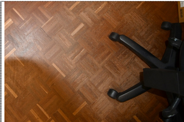
Figure 42. Typical damage to original floor where it is wearing in places where desk chairs are used. Fair condition.
