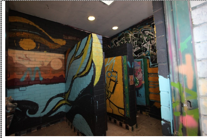
Figure 40. Interior view of later Toilet Block to the northeast of the Administration Building.
