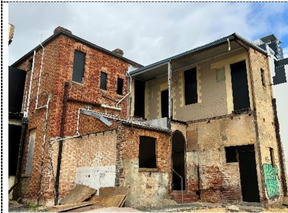
Figure 18. North and western elevations of Pearl Villa clearly showing vulnerable condition of the north elevation of Pearl Villa following the removal of non-original elements. Photograph: Hocking Heritage + Architecture, September 2023.
