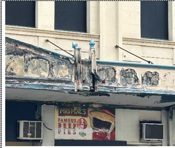
Figure 11. Damaged ornamentation to verandah canopy. Photograph: Hocking Heritage + Architecture, September 2023.
