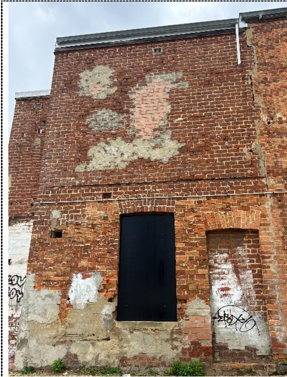
Figure 17. Upper storey addition to the south western end of Pearl Villa – contrasting brickwork. Photograph: Hocking Heritage + Architecture, September 2023.
