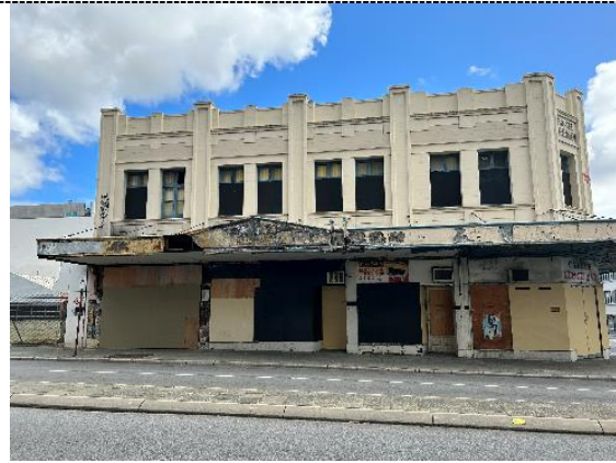
Figure 7. View of Hostel Milligan, Perth taken from east side of Milligan Street. Photograph: Hocking Heritage + Architecture, September 2023.
