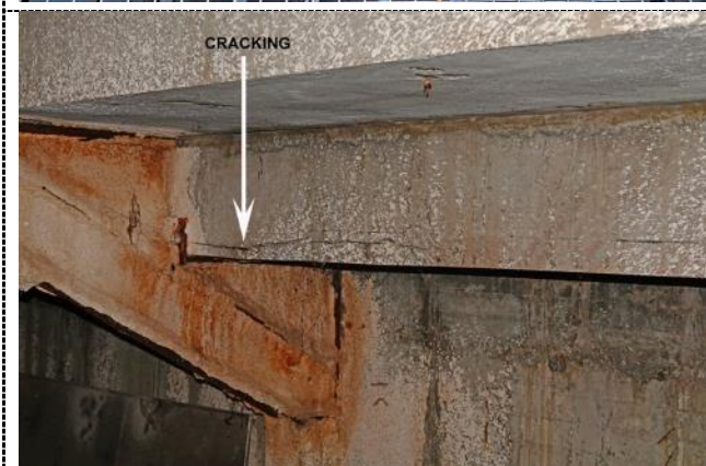
Figure 3. Velodrome grandstand – deterioration to lower concrete tiers
