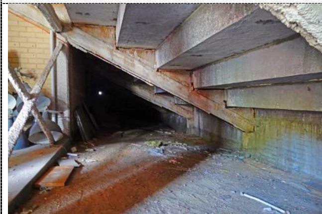
Figure 44. South-eastern undercroft A small section near the entrance door has been finished with a concrete floor and is used for storage. The remainder has a compacted earth floor.
