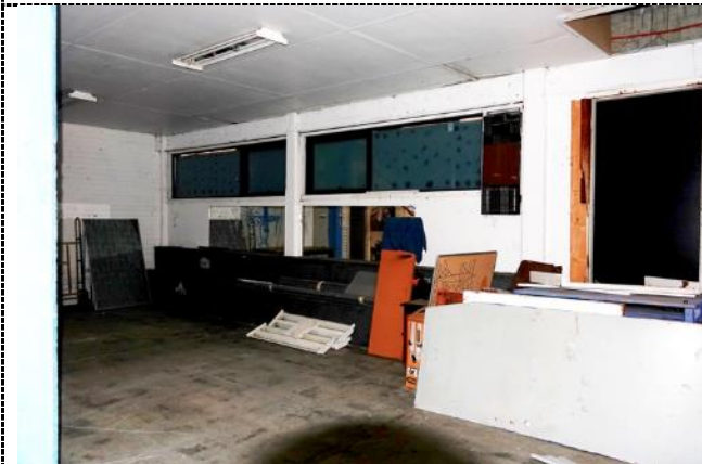
Figure 43. North-western undercroft – office/store – area below function room This area has basic finishes, which are not consistent with the original detailing to the rest of the building.
