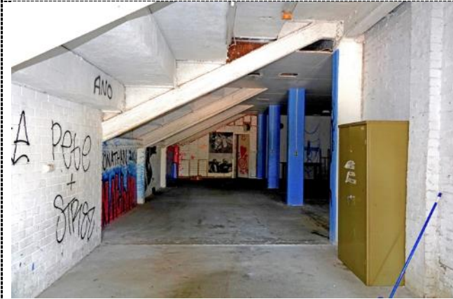
Figure 42. North-western undercroft – office/store – area below seating tiers The north-western undercroft area has been finished with a concrete floor, a mixture of painted and rendered walls, and a mixture of painted concrete and suspended ceilings. The finishes and detailing are consistent with a basic, post-construction fit out to make part of the undercroft habitable for an office, meeting room or similar function.
