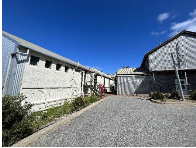
Figure 13. The north elevation presents in a single storey form with white painted brick finish. Windows are a mix of larger office windows with horizontal louvers and high level metal framed openings. This elevation does not contain any distinctive features.
