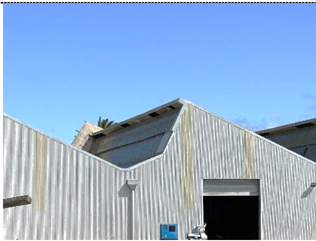
Figure 15. The glazed panelling to the southern side of the roof form and truck entry into the warehouse.
