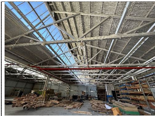
Figure 28. Saw tooth roof warehouse. The south facing saw tooth roof lights run the entire length of the bays in an east-west direction, facing south. The original glazing has been replaced with larger panels. 88
