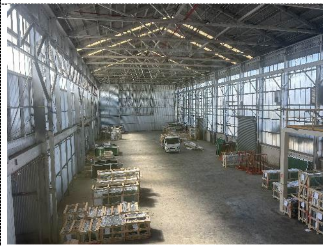
Figure 26. Southern warehouse, taken from the upper offices. The trusses are timber in the original section, while steel trusses have been used in the 1947 extension. The timber trusses have been painted silver.
