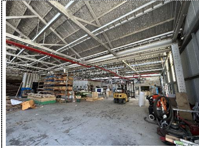
Figure 29. Saw tooth roof warehouse. The remaining warehouse bays date to the original 1930 construction, with timber trusses throughout. The timber has been painted silver.
