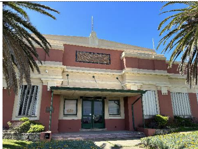
Figure 9. The main entrance is marked by a simple and stripped back cantilevered canopy, attached to the facade by structural tie rods. The entry element stands proud to the façade with decorative parapet, pilasters and horizontal pressed cement banding.
