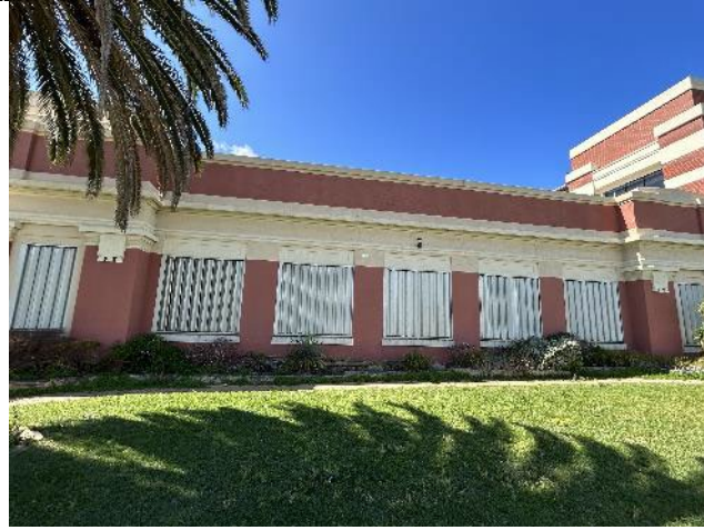
Figure 10. Providing a counterbalance to the dominant factory frontage, the single storey office building has a horizontal emphasis with a symmetrical presentation. The central entrance section is flanked by recessed wings which present with a rhythm of fenestration.
